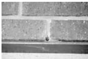
Figure 15-36 Small plastic weep tubes are not recommended because they clog too easily both during and after construction.
