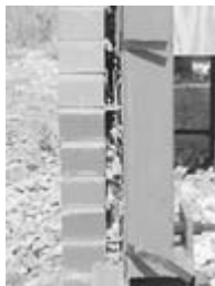
Figure 15-38 Use of a proprietary drainage mat does not eliminate the need for proper construction procedures to minimize mortar droppings.
