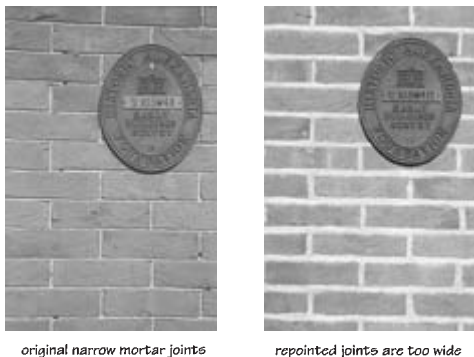
Figure 16-10 Original (left) and repointed (right) halves of building have very different appearance.
