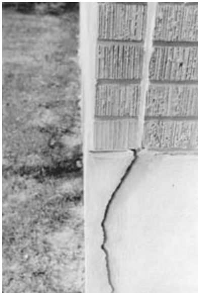
Figure 9-20 Brick expansion forces may exceed tensile strength of concrete. (Photo courtesy BIA.)
