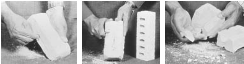
Figure 3-31 Under-burned bricks are easily scratched or scored with a coin, cut with a knife, or broken by hand. (Photos courtesy Brick Institute of Texas.)
