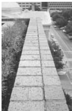
Figure 9-51 Brick rowlock copings have a high probability of cracking.
