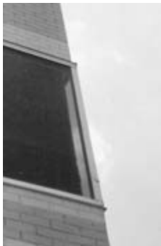
Figure 9-40 Protruding window invites leaks at head.
