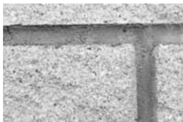
rough surface, bond line separations
