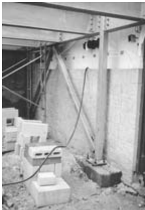
Figure 18-3 Garden hose placed briefly in wall cavity to test for obstruction of water flow to weeps.
