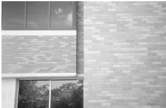
Figure 15-22 Raked horizontal joints in the wall panel on the left give the masonry a darker appearance than the concave tooled joints in the wall panel on the right.
