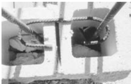
Figure 15-48 Mortar protrusions into the wall cavity or unit cores will inhibit the flow of grout and create voids within the section.
