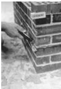
Figure 15-30 Trim flexible flashing flush with outside face of wall. (Photo courtesy BIA.)
