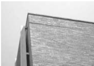
Figure 9-7 Parapets can expand and contract at a different rate than the building walls below.
