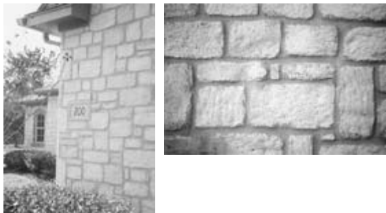
Figure 4-3 Simulated stone made to resemble natural rubble stone is not the same strength and quality as architectural cast stone.
