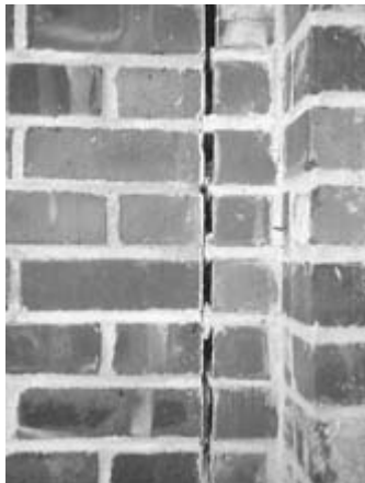
Figure 9-14 Mortar bridges across an expansion joint can cause localized spalling where movement is restricted.
