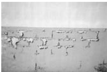
delamination of exterior coating
