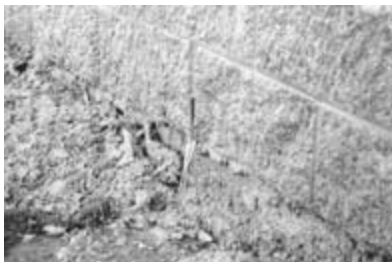
Figure 18-4 Water should drain immediately and freely from the weep hole immediately below the test location.
