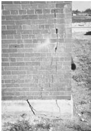
Figure 9-6 Opposing moisture expansion of brick and curing shrinkage of concrete slab can cause cracking at building corners if differential movement is not accommodated.
