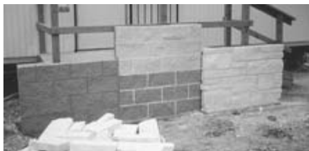
Figure 17-4 Traditional masonry sample panels for evaluating unit color, color range, mortar color, joint tooling, and general workmanship.
