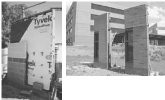
Figure 17-5 Masonry mock-ups should include all elements important to the performance and appearance of the masonry such as backing wall, anchors, drainage mat, flashing, weeps, movement joints, and windows.
